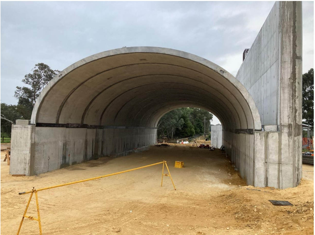
Figure 17 Legacy Initiative - Underpass 9527 under construction to facilitate future bridle path and PSP
